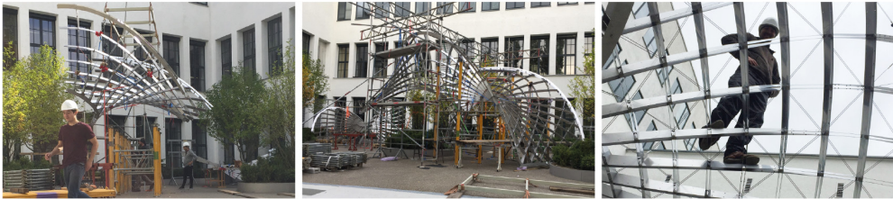
Figure 14: Installation on site. The prefabricated segments of up to 400 kg, were positioned with a crane, temporarily supported, and bolted together by hand. To activate the structural behavior of a gridshell, the completed grid is braced diagonally and fixed at supports in vertical and horizontal direction. (Images: Andrea Schmidt)
